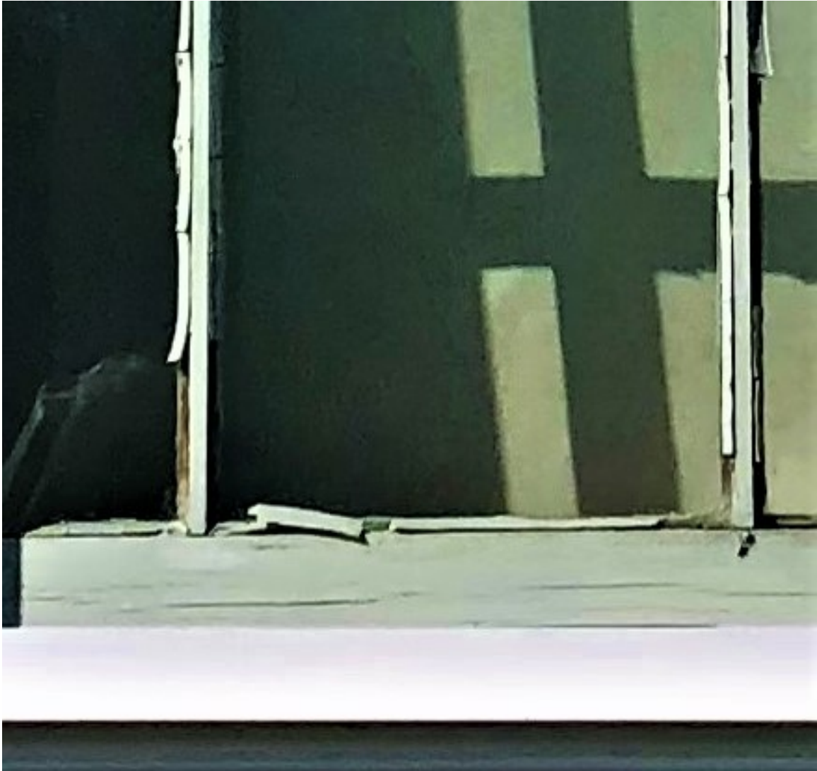
Photo 1. Close view of deteriorated window sashes. The east facing windows have shown extreme wear for several years. Several panes of glass are slipping out of the seam.
