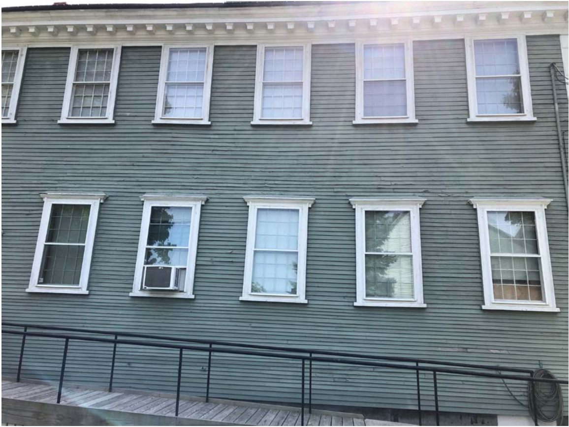
Photo 2. View of west side of museum. Window headers show severe deterioration and wood rot. Tin/aluminum covers are planned to match front facing window restoration work completed during the 2013 museum roof and cupola restoration work.
