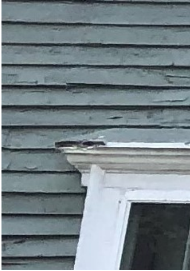
Photo 3. Close up of west facing window with damage wood rot and the beginning of water seepage into window frame.
